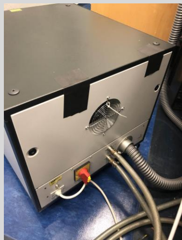
Laser Chiller in 66-427 Showing Connected Water Hoses
