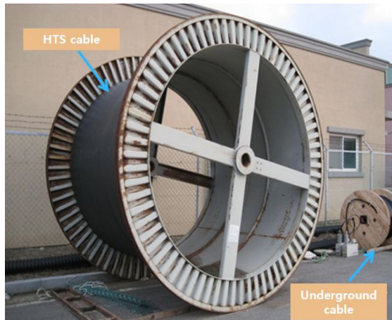
34.5 kV HTS cable*
